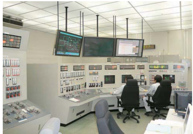
HTTR Central Control Room
