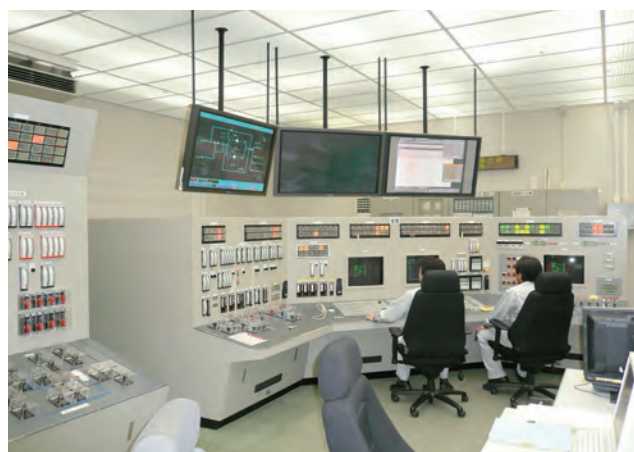
HTTR Central Control Room
