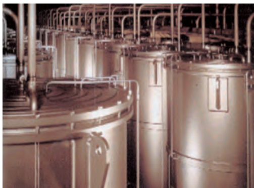
(a) Uranium enrichment plant
