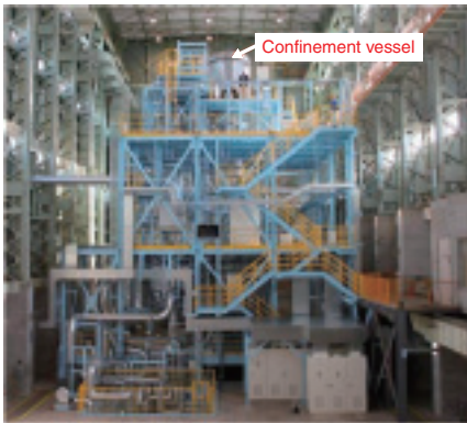
Fig.3-27 IFMIF/EVEDA Li Test Loop (ELTL) after completion of construction The ELTL, which holds 2.5 ton Li, comprises three floors whose width and depth are 15 m each. The total height of the ELTL is 20 m, and a test section called TA is installed at the top of the confinement vessel.
