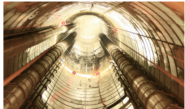
Fig.12-27 View from inside of the Main Shaft: upward perspective Main Shaft diameter is 6.5 m.
