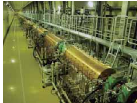
Fig.5-1 Annular-ring coupled structure (ACS) cavities installed at the downstream of Linac
