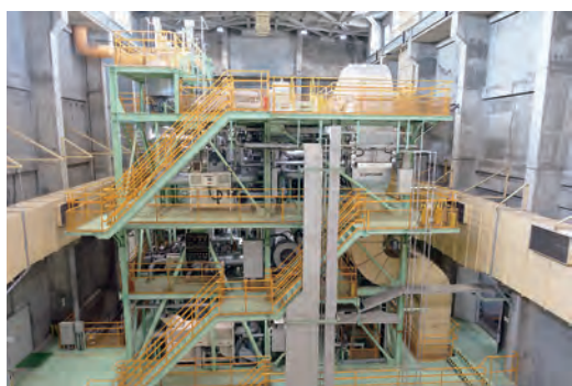
Fig.7-2 Plant-dynamics test loop
